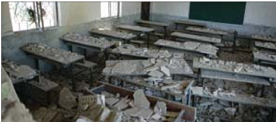
Marines with Civil Affairs Detachment 4-4, Regimental Combat Team 1, 1st Marine Division assess the damages of the Hareery School in Fallujah, Iraq, Feb. 14, so the rebuilding process can begin.
